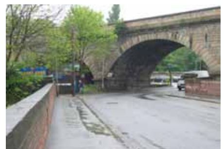
The railway viaduct arch over Canal Road is the gateway to Armley from the north.
