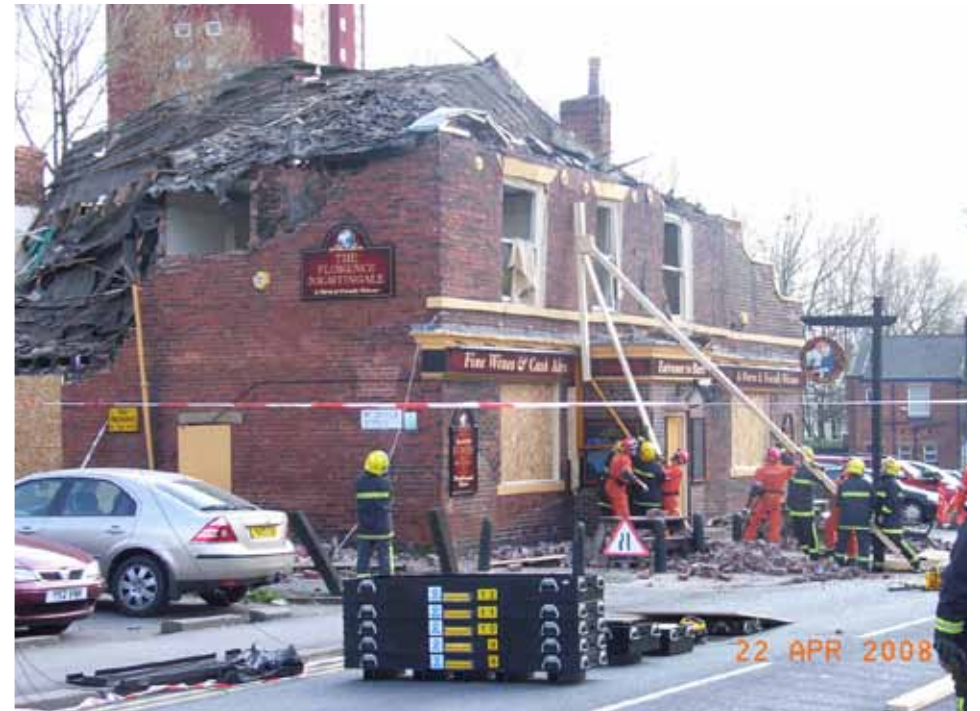
Figure 2. This is another gas explosion that occurred at the Florence Nightingale Pub opposite St James's Hospital. The pub had been vacant for several months and the explosion is thought to have occurred due to someone attempting to steal the cooker. Building Control worked closely with the Emergency Services to carry out controlled demolition and allow the Fire and Rescue Team and SOCO access to assess the site.
