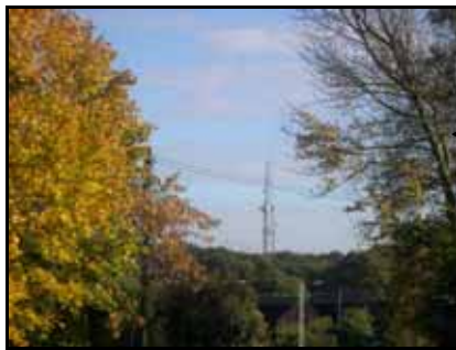
Macrocell base station comprising a 45m lattice tower capable of accommodating 65 antennas
