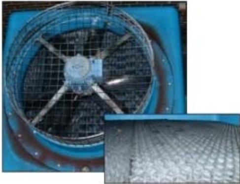
Above: The cooling towers in wet air-conditioning systems need to be treated regularly to prevent Legionella.
