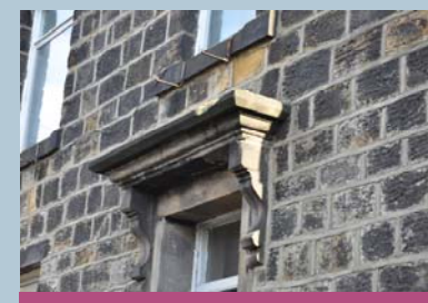
Porch with stone corbels creating an active frontage to this side gable.
