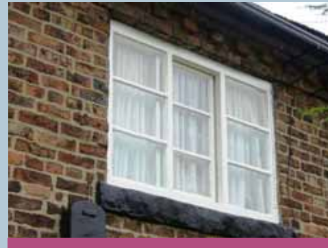
Horizontal sliding or Yorkshire sashes are a local window detail of interest
